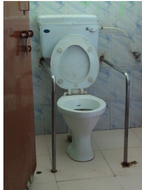
Toilet for disabled children at Chingari Trust Rehabilitation Center, Bhopal, Madhya Pradesh, India, 2017, photo by Lewis Koch
